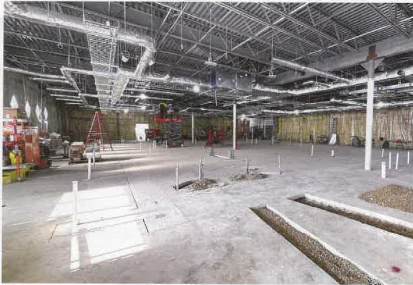
The build out of the Clinic's new Urgent Care, shown here at an early stage, entailed a "to-the-studs" redevelopment. | CUSTAR
